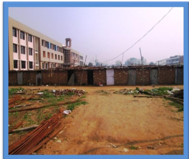
Construction Labour: Missing Basic Amenities
